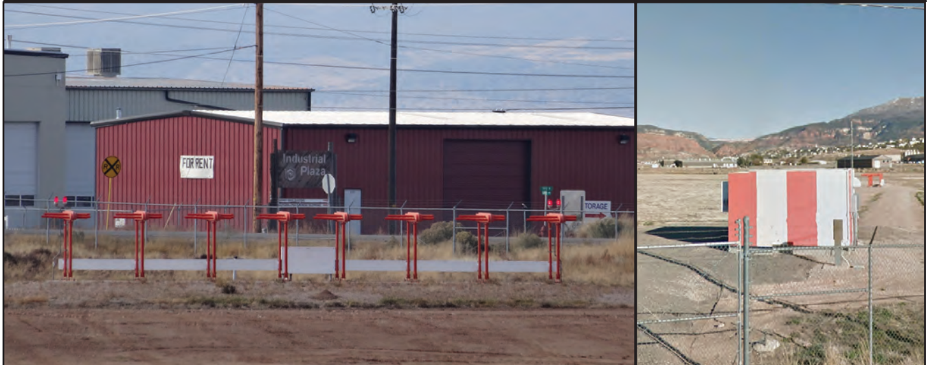
Figure 3.22 Localizer and Electrical Vault (1)
