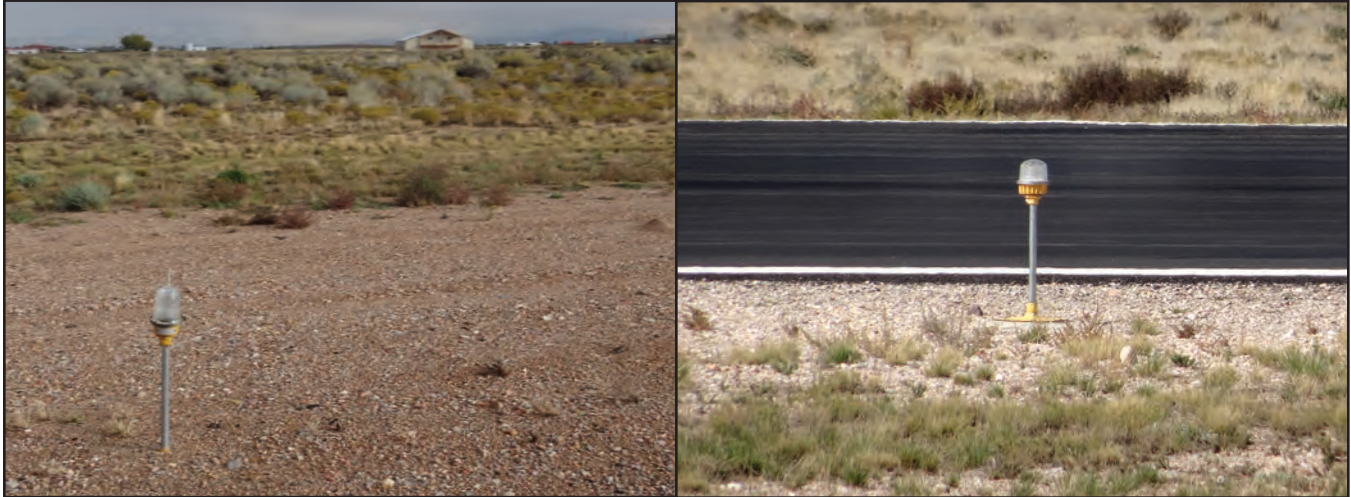
Figure 3.28 Medium and High Intensity Runway Edge Lighting (7 and 8)
